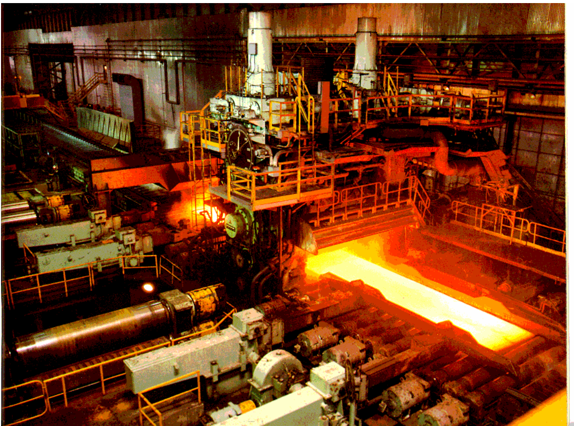
Figure 1: Picture of COSIPA's 4100 mm plate mill.
